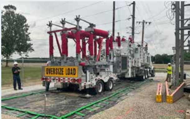
Mobile Substation being delivered from Wabash Valley.
